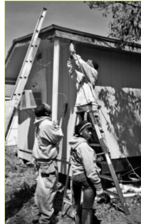
YouthBuild students, Confessor Santa III, Bessie Williams, and Justin Schanck, work on a home damaged by Hurricane Katrina.
