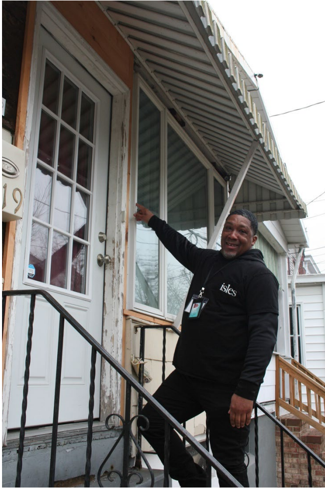
Lead Hazard Control Specialist, Bennett Sims pointing out the difference between the previous framing around the door and the new door and windows that the Isles team replaced.
