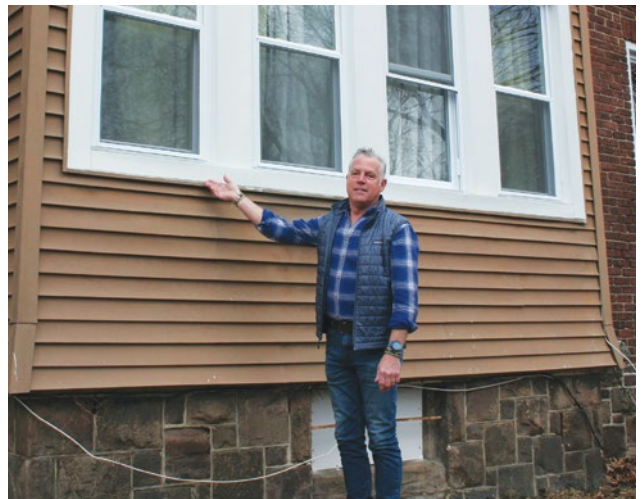
Lead Hazard Construction Manager Ron Voorhees shows the windows, doors, and framing that we replaced on this home due to lead paint dust as compared with the stairs that tested negative for lead.
